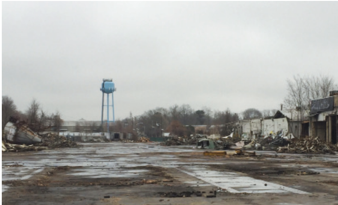
Photograph of nearly demolished Art Color property. This part of the project should be done by late Spring. Next steps are to install infrastructure and begin the building process.
